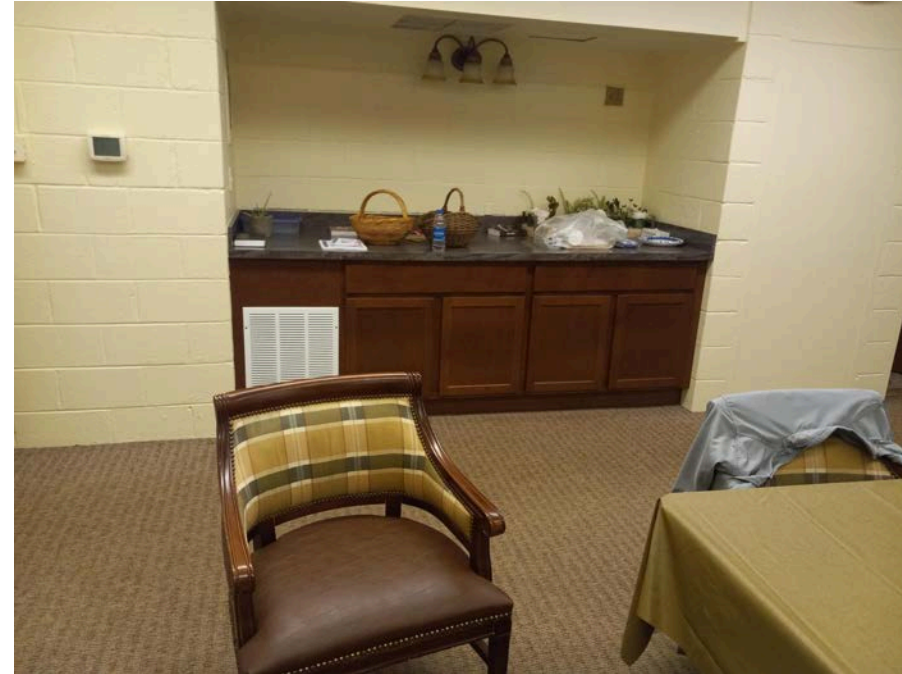
Mold started in this sink area
