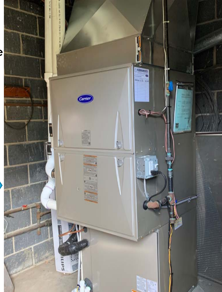
CS/COI HVAC → Repairs/Replace
