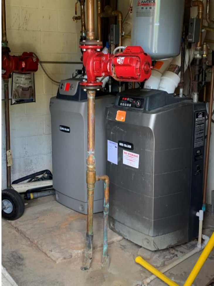
← Church Boiler- Repairs/Replace
